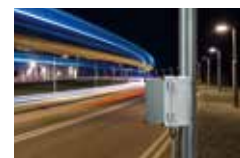
Street lighting control
